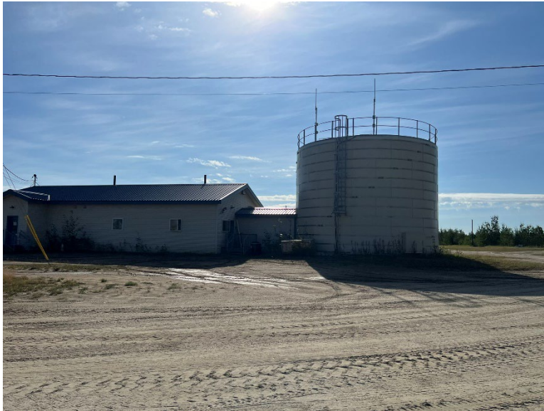
FIGURE 10 HUSLIA WATER PLANT
