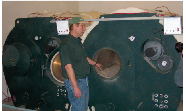
Dual Garn WHS boilers in Tanana. Photo Courtesy of AEA
