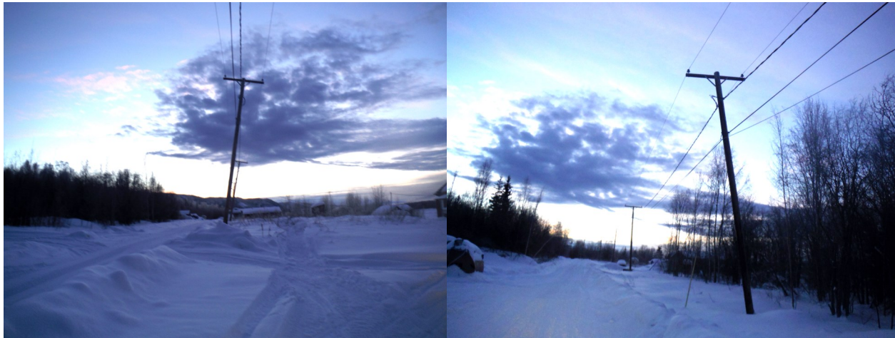
Rampart Leaning Power Poles. 2014
